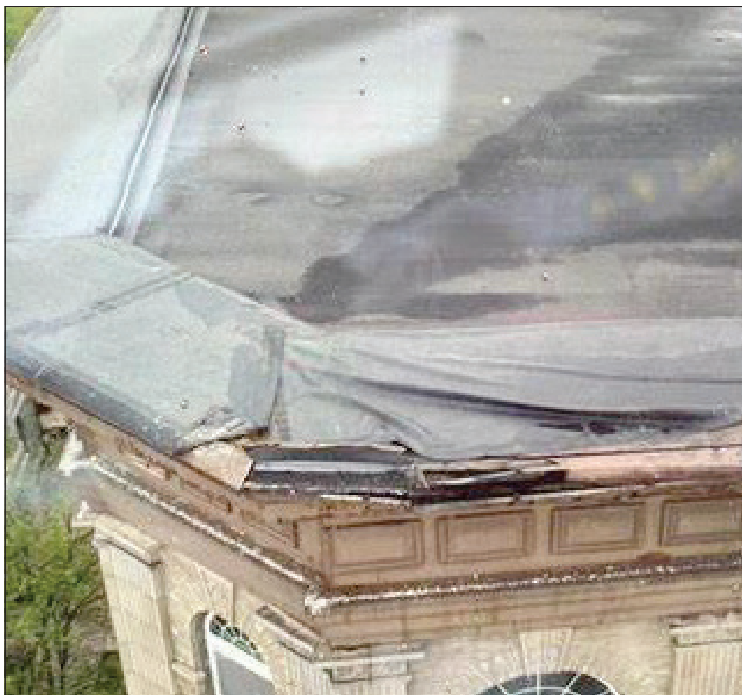
A drone image of the roof of a 276 High St. building shows a damaged roof. Parts of the roof collapsed Tuesday morning. The Holyoke Fire Department continues to investigate the building, which is located next to City Hall.
