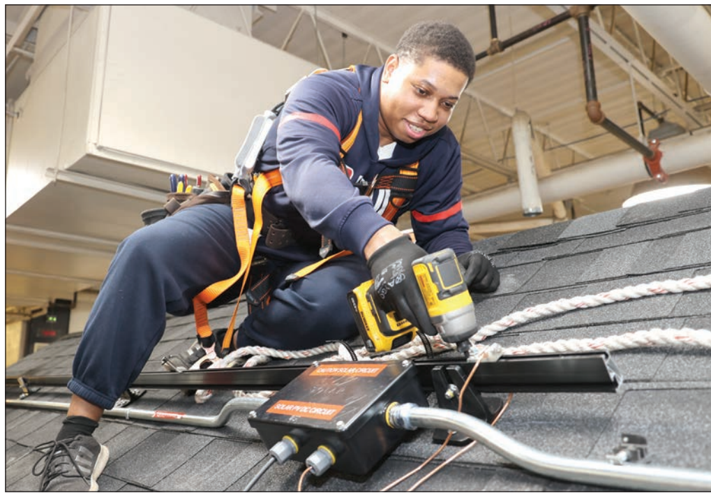
Jayshawn Brown, a student in HCC’s solar tech training program, works on a solar panel installation project at Dean Technical High School.
